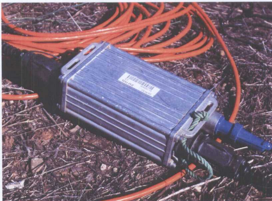
Line power unit and Telemetric station Unit SN 388 UL1
